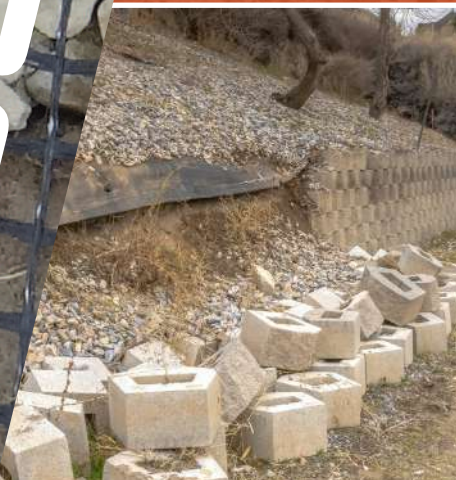
WITH NO GEOGRID INSTALLED
