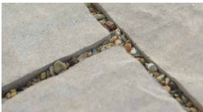
Special materials are used in the joints and in the permeable base below, to encourage water to flow through.
